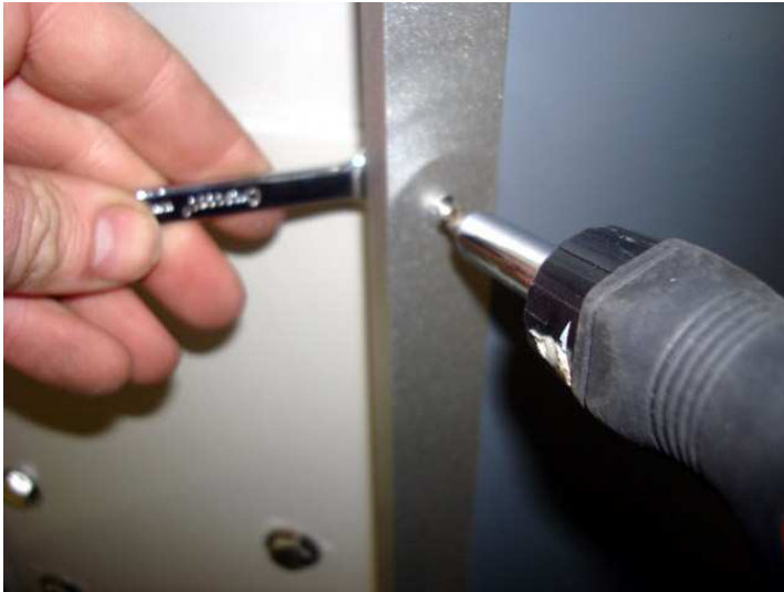
Notice clean crisp joint with seal inside. Above and below
