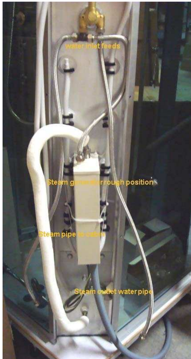
Typical plumbing set up
